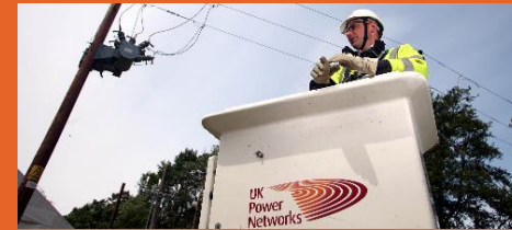
Photo: UK Power Networks
