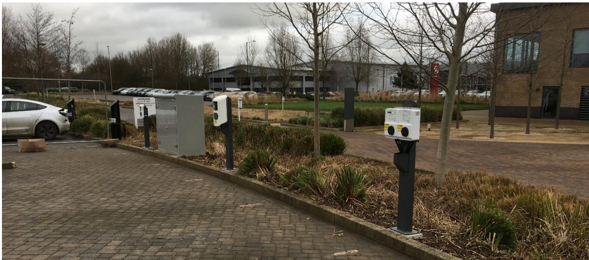
Figure 8 – FAT site at HCVS Trowbridge, showing the Swarco CP to the right and Alfen CPs either side of the grey distribution cabinet
