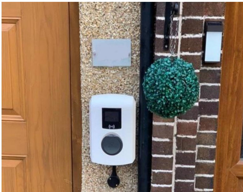
Figure 2 – EV CP installed at a British Gas driver's home by Centrica
