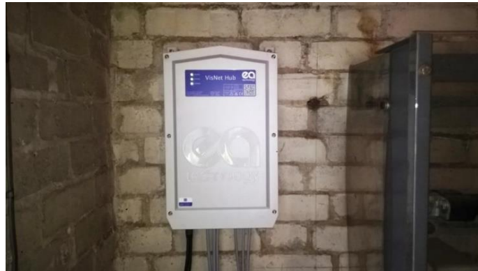
Figure 20 – VisNet Hub installed at Whitechapel Rd GPO Parcels substation
