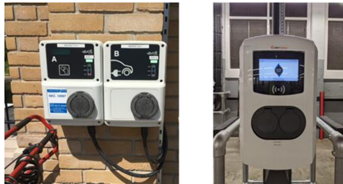
Figure 5 – Charging infrastructure at Royal Mail depots (existing CP, left; newly installed CP, right)
