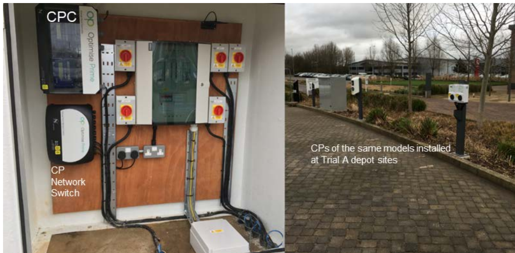
Figure 5 – CPC and CPs at test site, replicating depot installations
