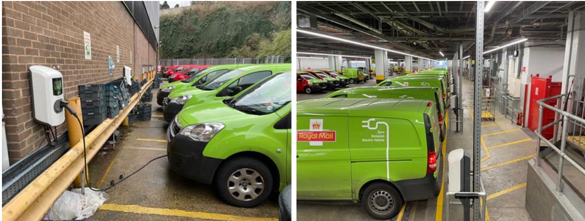
Figure 4 – Royal Mail EVs charging at Dartford Delivery Office (left) and Mount Pleasant Mail Centre (right)
