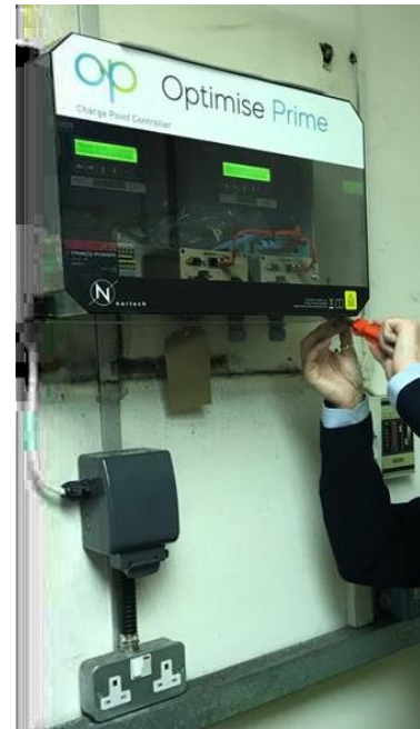
Figure 2 – WS2 Charge point controller
